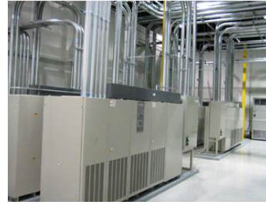
UPS battery room
