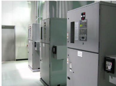
three-phase power transfer switches
